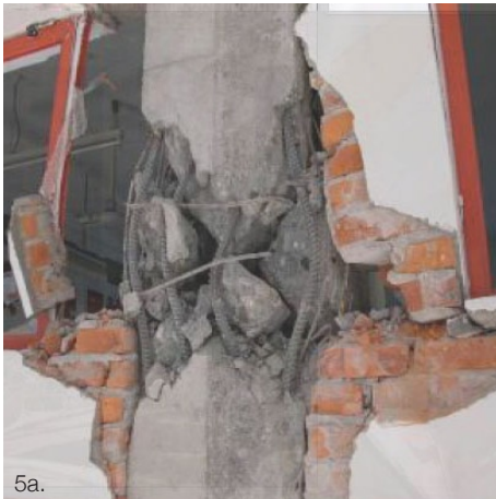
Figure 6 a & b. Collapse of apartment in 512 Sichuan Earthquake [10]
